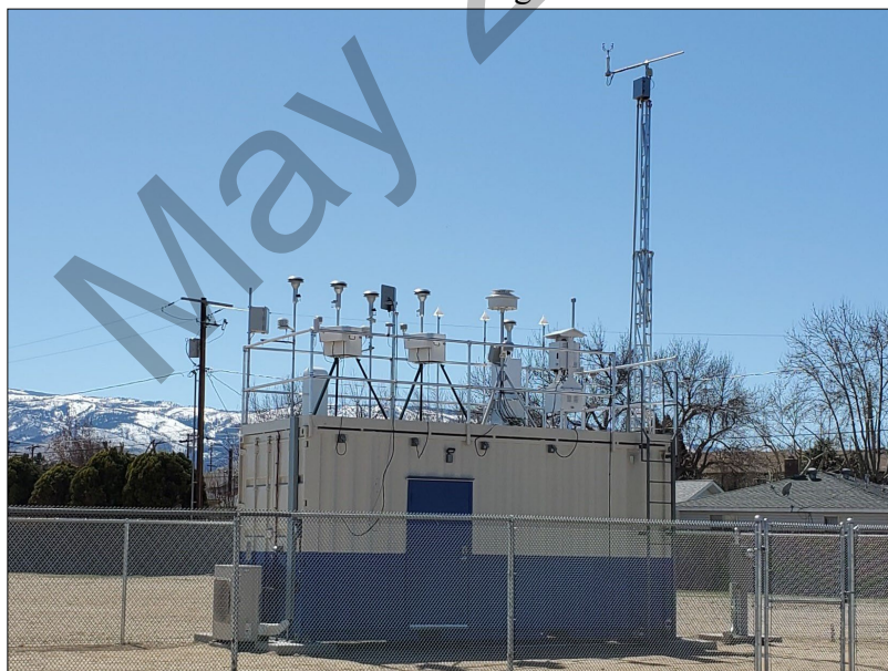
Figure 8 Reno4 Monitoring Station
