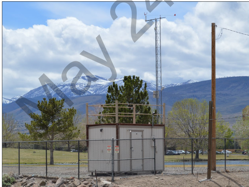
Figure 10 South Reno Monitoring Station
